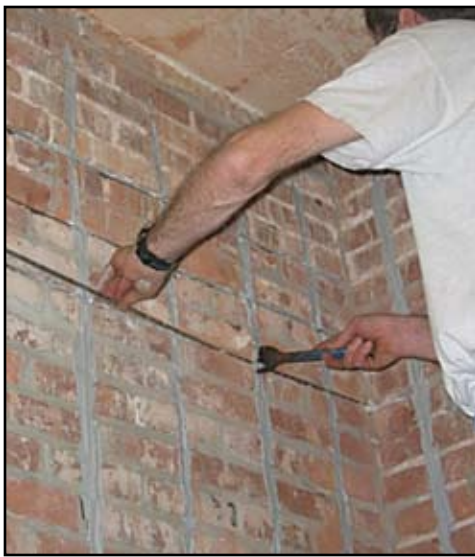
Figure 3: Crack stitching of a brick wall with NSM CFRP Bars in Boston, MA. The wall was severely cracked due to foundation settlement.
