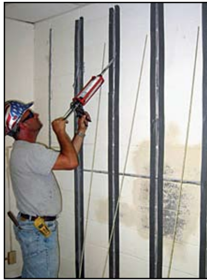
Figure 1: Flexural strengthening with NSM GFRP Bars of a CMU wall in Kansas City, MO. The wall was damaged due to lateral displacement. Note the repaired crack at mid-height.
