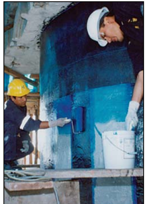
Figure 4: Strengthening with CFRP laminates of a 17 th century masonry cathedral tower in Peru. Vertical reinforcement provides flexural strength. Hoop reinforcement provides confinement to restrain lateral expansion under earthquake forces.
