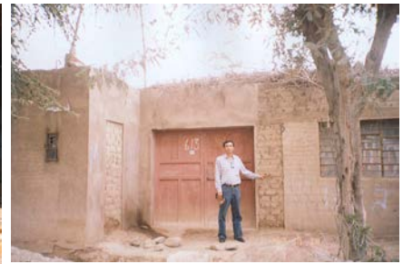
Figure 21: Demonstration house with partial reinforcement in Parcona, Ica. This is the station of the Peruvian Geophysical Institute, in which a peak acceleration of 0.49g was recorded.
