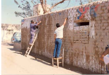
Fig. 24: Reinforcement of existing house of Fig. 19 in Ica, in 1998. Workers mark position for horizontal strip.
