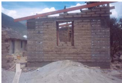
Fig. 31: Strips of wire mesh nailed to the corners, and wood collar beam.
