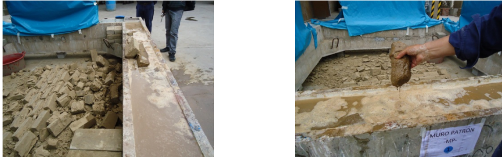
Figure 9: Overturned wall TW1 and condition of the adobes in the base.
