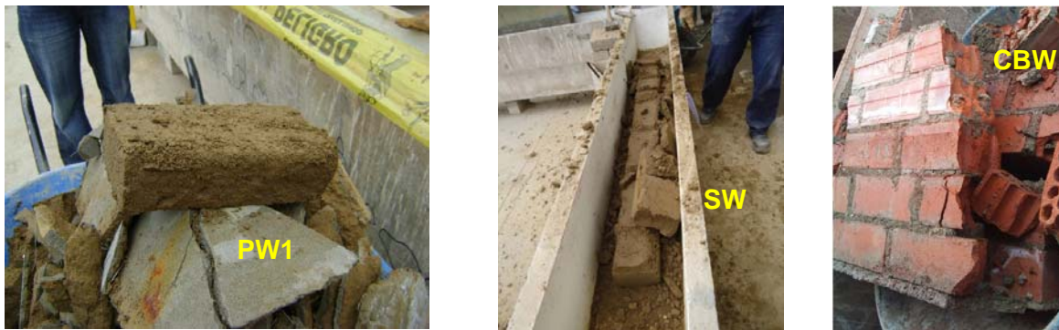
Figure 12: Inspection of masonry units in the base after demolition of the walls.
