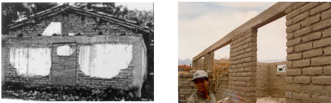
Figure 2: Good behavior of one-story adobe houses confined by RC elements, Ometepec Mexico [4] (left) and Nasca Peru [5] (right)
