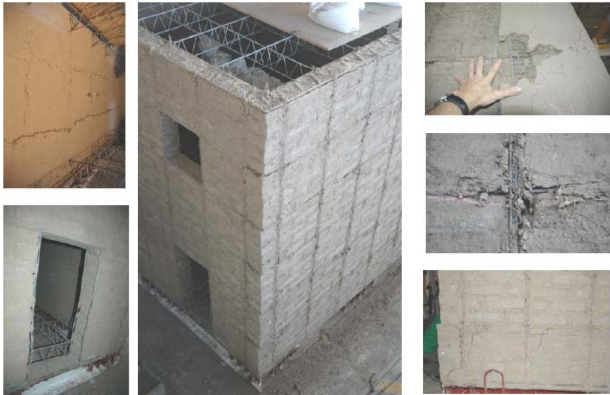
Fig. 7: Damages pictures before 4º Test (130 mm); Left a) Indoor; b) Entry; Center c) Sides without rendering, Right d) Detachment of rendering; e) Double truss-type prefabricated f) Cracks wall.
